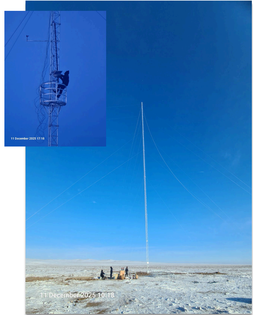
Recently Installed 120m Wind Mast
